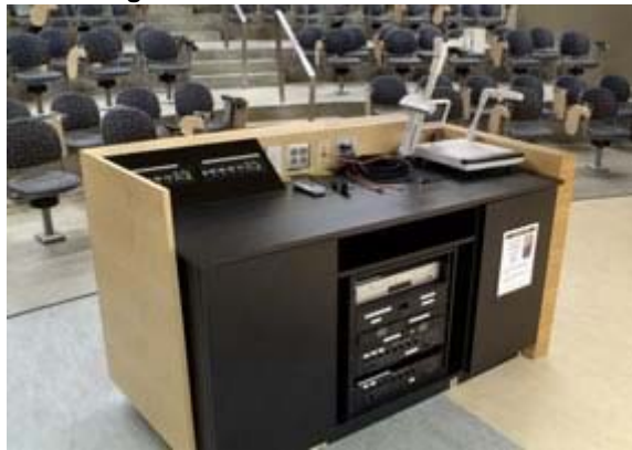
Figure 7. Instructor's Control Station
